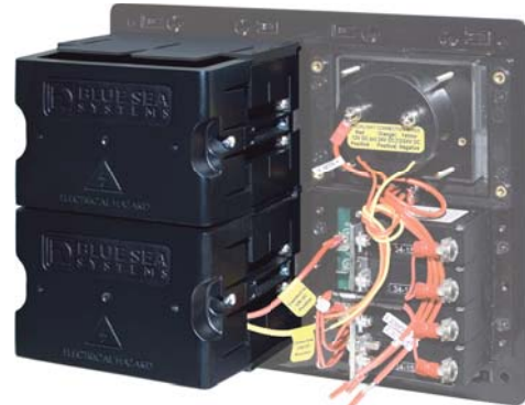
1341 installed on an AC/DC Panel
