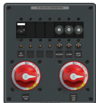
Traditional Metal Battery Management Panels
