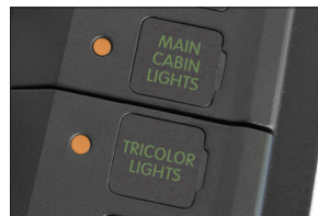
Backlit labels aid circuit identification in low light conditions
